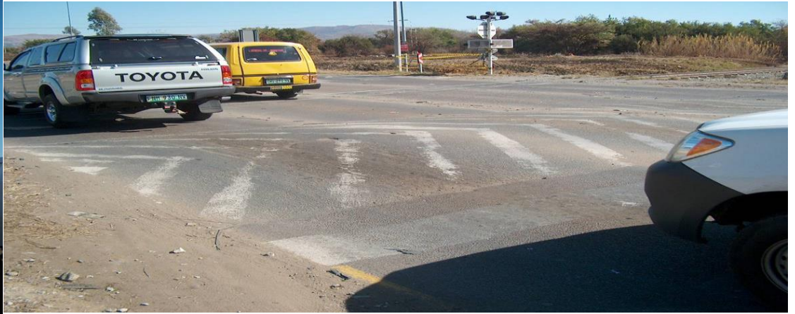
Clear Road Surface Speed Hump
